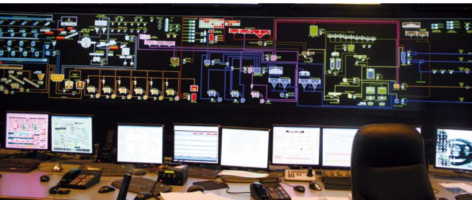
Control room at the Clarabelle Mill at Vale Inco's Sudbury operations.
