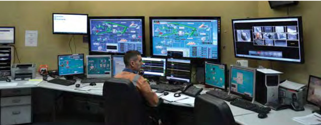
Processing control room at the Savage River mine, Tasmania.
